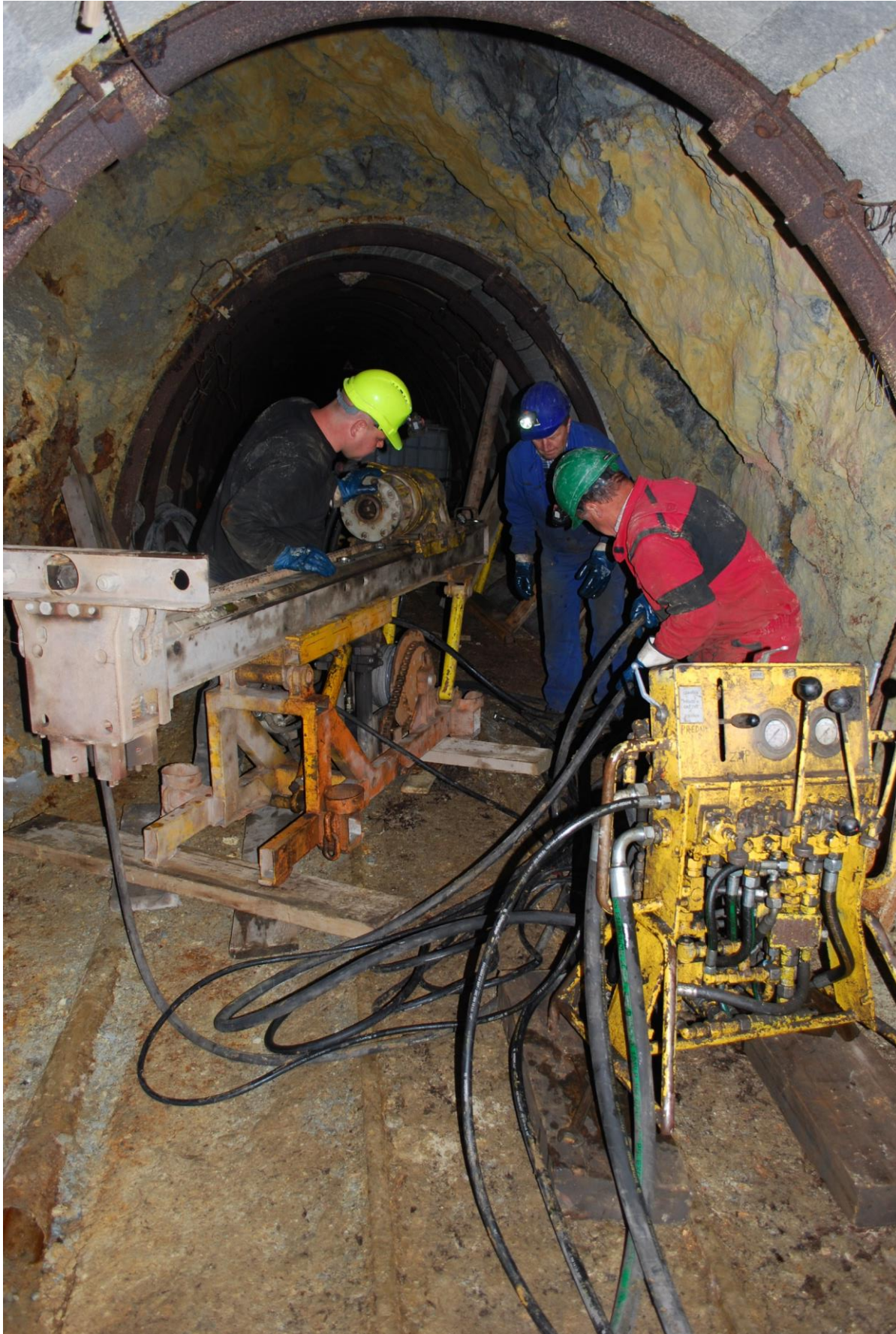
Image 4: Drill rig and ancillary equipment being set up at the drill site within the underground Andrej adit
